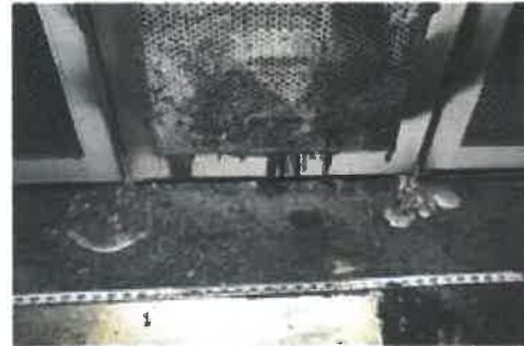
Figure A.1: Photograph taken during decommissioning of the BESS shows a pool of molten aluminium on the floor in front of Rack 15 [ 11].
