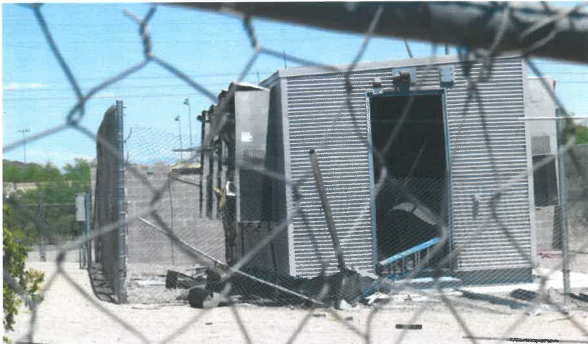
Figure 4: The 2 MWh McMicken (Arizona) BESS after the explosion on 19 April 2019
